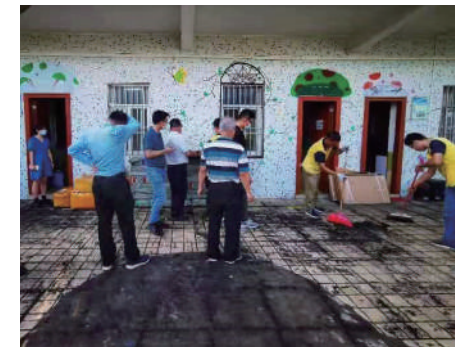
Cleaning and removal of old and obsolete equipment and facilities at a kindergarten in Dongsheng Island
